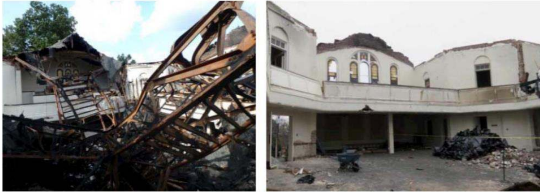
FIGURE 1.—Site photos of initial damage scan and after demolition scan areas.
