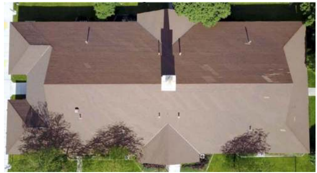
ILLUSTRATION 4.—Initial Image at 180 Feet to See Defect Zones
